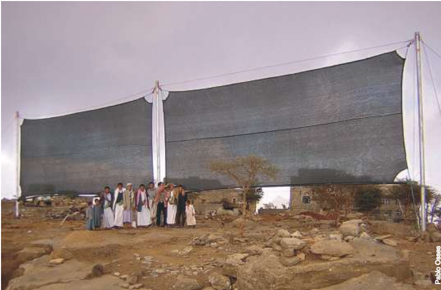
The team that constructed the LFCs, from FogQuest, ICS, and the villages
