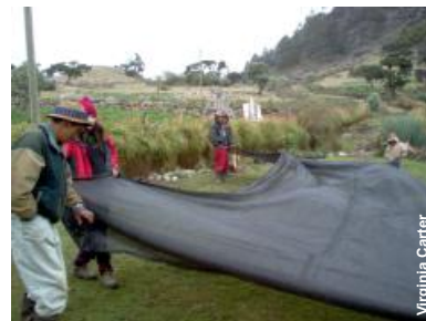
The mesh being sewn onto the support cables for the LFCs in La Ventosa.
