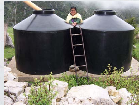
Fog water is stored in clean tanks for village use.
